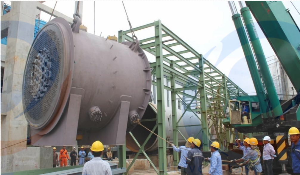
90 Ton Boiler & 70 Ton Stack at WSA Plant South Pasific Viscose Purwakarta
